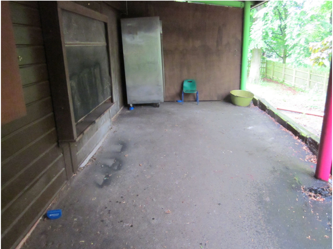
Photo 2: View of area of to back of the building to be infilled.
